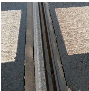
State of the art: Damage caused by detached joint material
